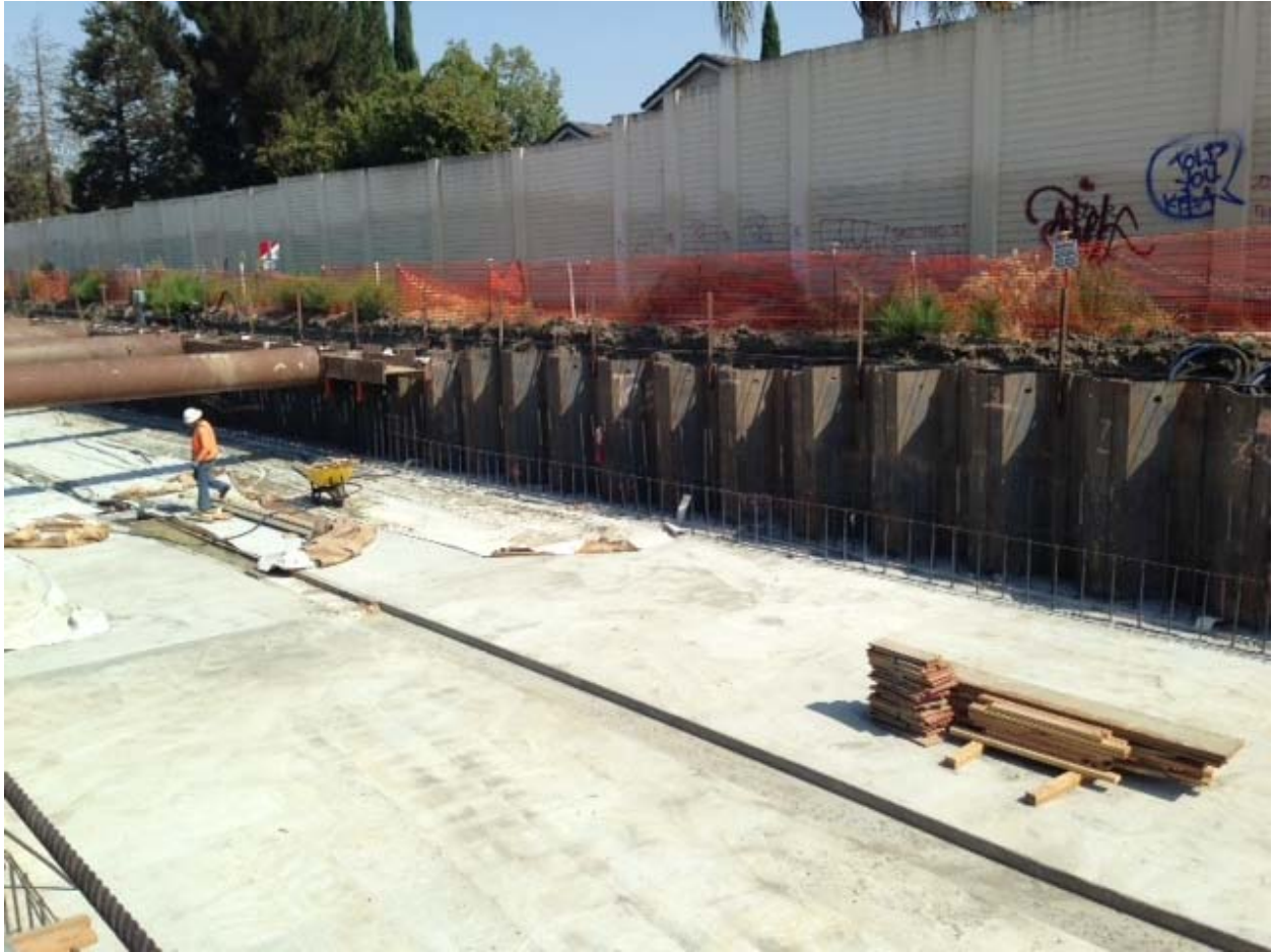
Another location where impalement protection is not provided. Concrete Masons were exposed to unprotected vertical rebar during the casting of this section of slab.
