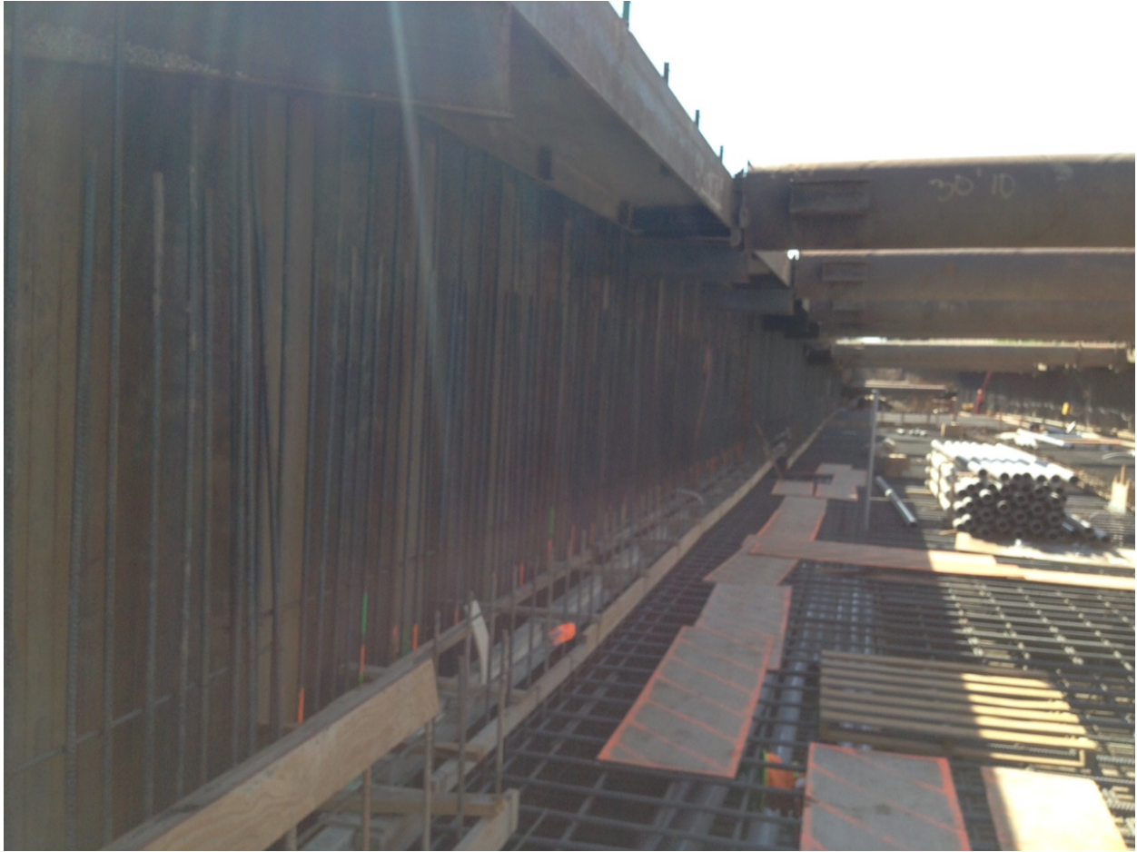
Another work area on the project where impalement protection has not been installed next to a temporary walkway.
