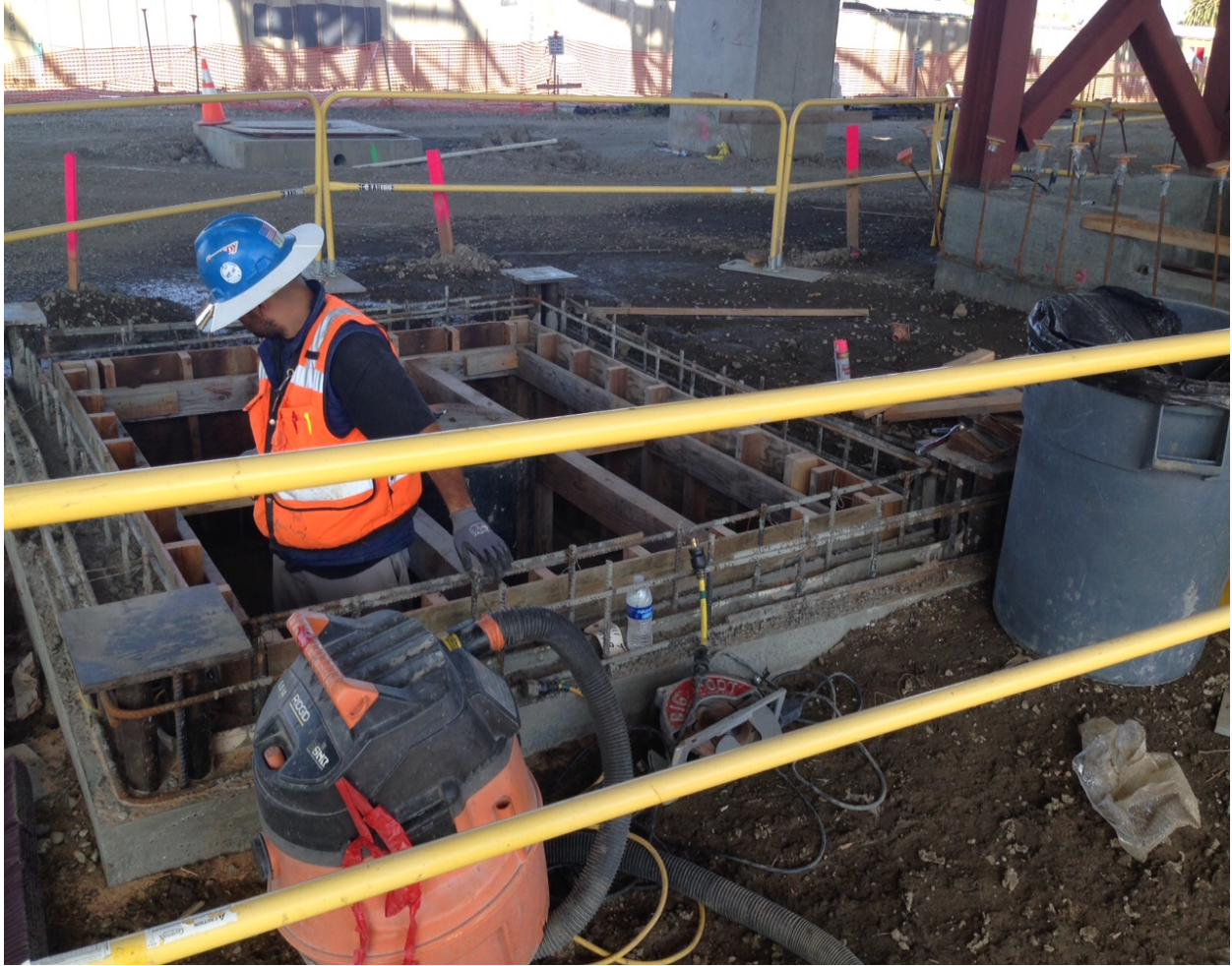
The worker in the photo is exposed to unprotected vertical rebars
