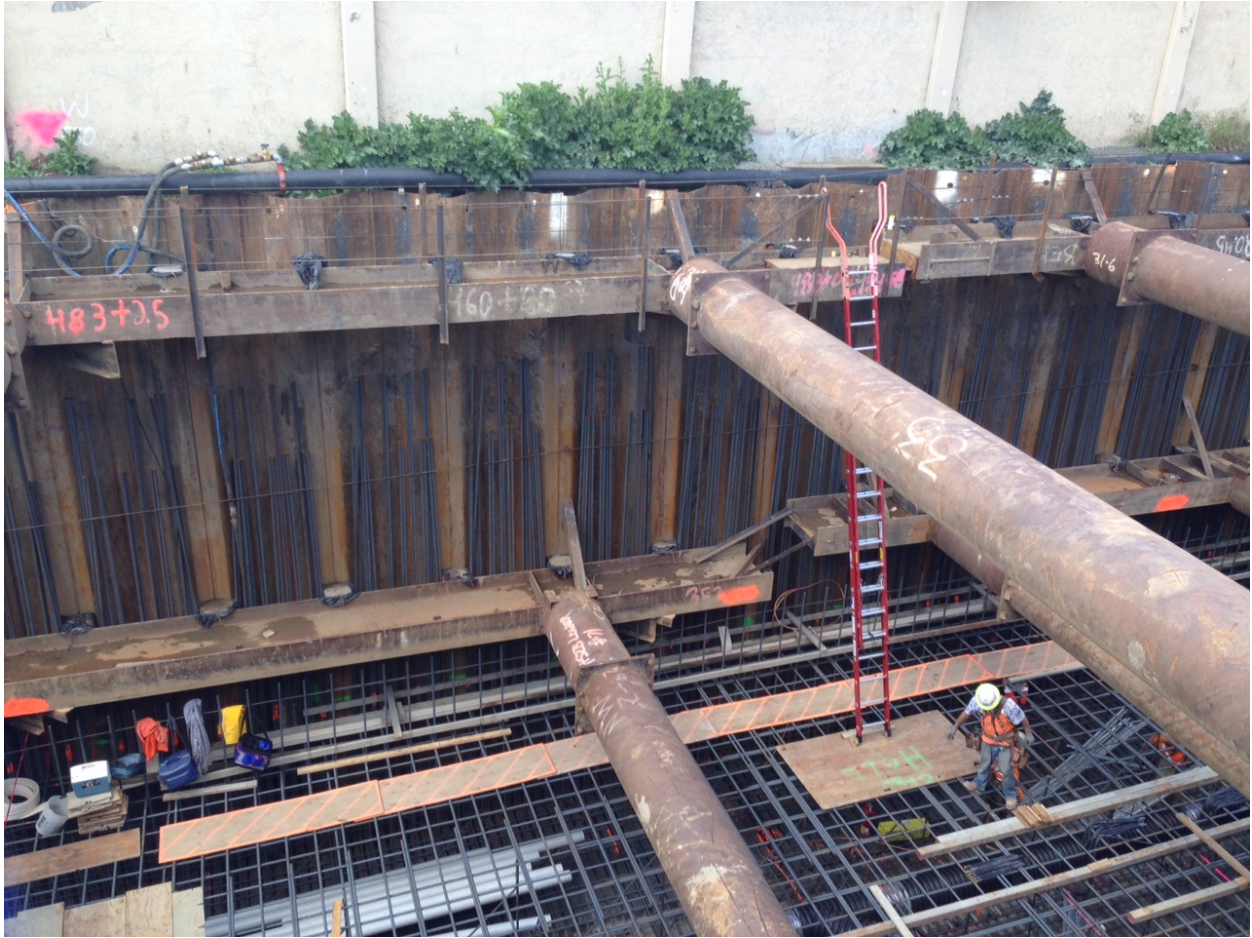
Unprotected vertical rebar next to an active temporary walkway
