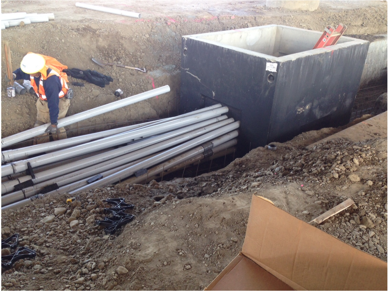
The underground electrical crew is exposed to impalement during the installation of underground electrical system.
