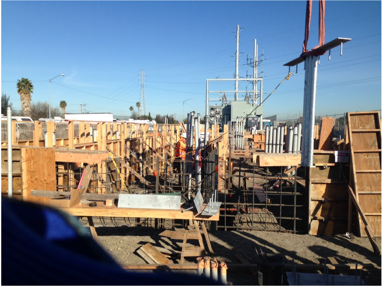
Workers are only partially protecting vertical rebars in the active work area.
